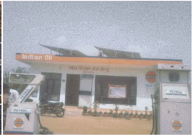
Sewa Kendra(Petrol Pump), Meerut. (5 KW Roof Top Solar Power Plant)
