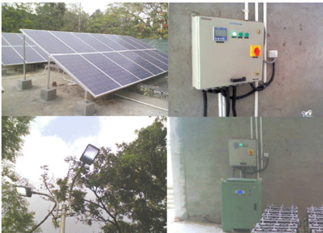
Raj-Bhavan, Ranchi, Jharkhand. (10 KW Roof Top Solar Power Plant)
