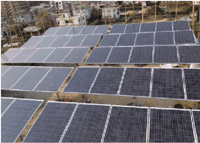
Lucent Publications, Patna (60 KW Roof Top Solar Power Plant)
